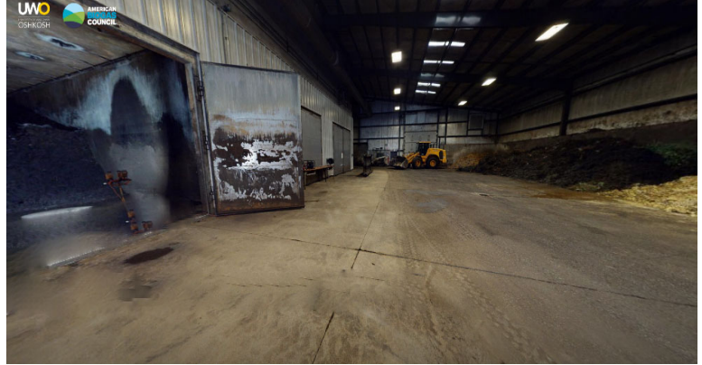
On the right: view of the feedstock receiving & mixing bay area. On the left: view of the digester chambers
