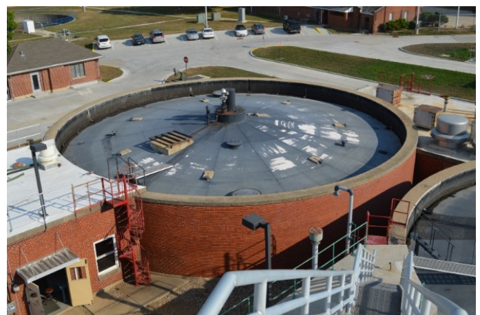
One of four anaerobic digesters, aerial view
