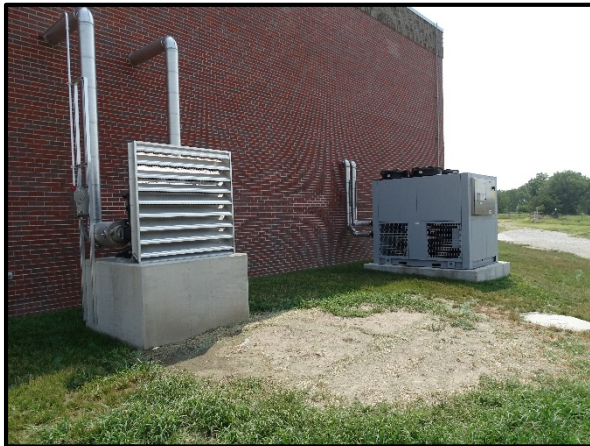
Heat Exchanger/Glycol Chiller
