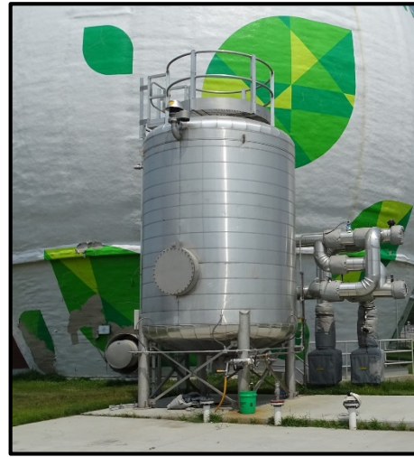
Hydrogen Sulfide Removal
