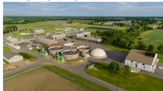
Digester Complex with two CHP Units Source: St Cloud NEW Recovery Facility
